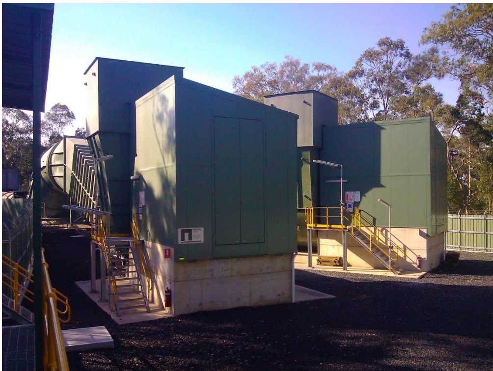
Plate 7.18: Chain Valley main ventilation fans
